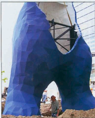
This view of the assembled and installed right and left legs reveals the bear's internal steel superstructure and shows the flange created to facilitate bolting of the bear's body parts at their seams.
