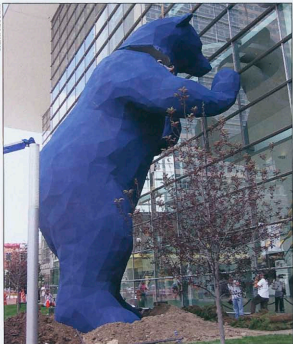
The Kreyler & Assoc. installation crew lowers the head into place on artist Lawrence Argent's bear sculpture. Commissioned for the Colorado Convention Center, it bears the apt title, "I See What You Mean."
